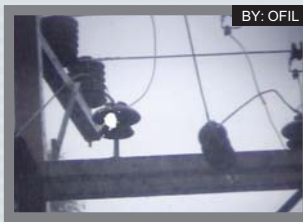
Arcing from a defective pin-and-cap insulator.
