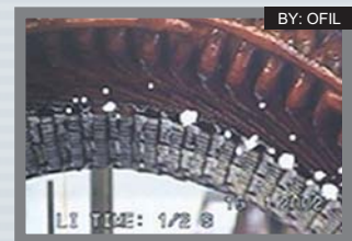
Motor 6.6 kV, 2500 HP after repair: 14,000 pC at 3.8 kV. Coil was sent for rewinding.
