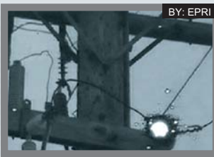
Arcing from a 23.4 kV porcelain insulator.
