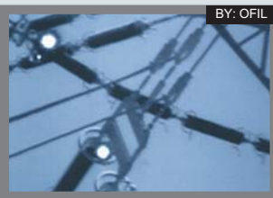
Improperly installed corona ring.
