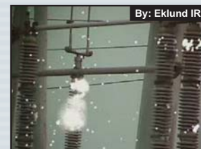
live flashover captured by the DayCor®II
