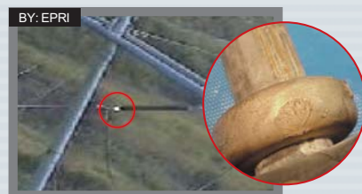
Damaged polymer insulator.
