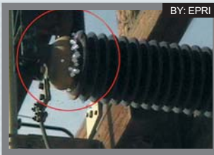
Arcing from the cap of substation post insulator.
